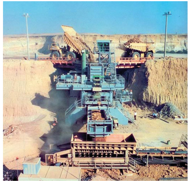
Fig. 2. Two-point stationary crushing reloading station [6]
